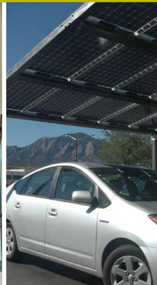
Carport: 2.85kW Lumos Solarscape Carport by Lighthouse Solar Boulder, CO
